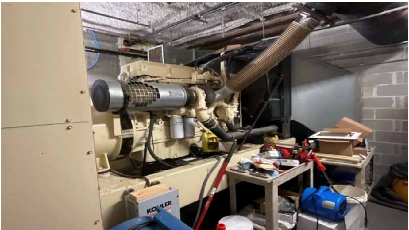
Condo Bldg Generator
