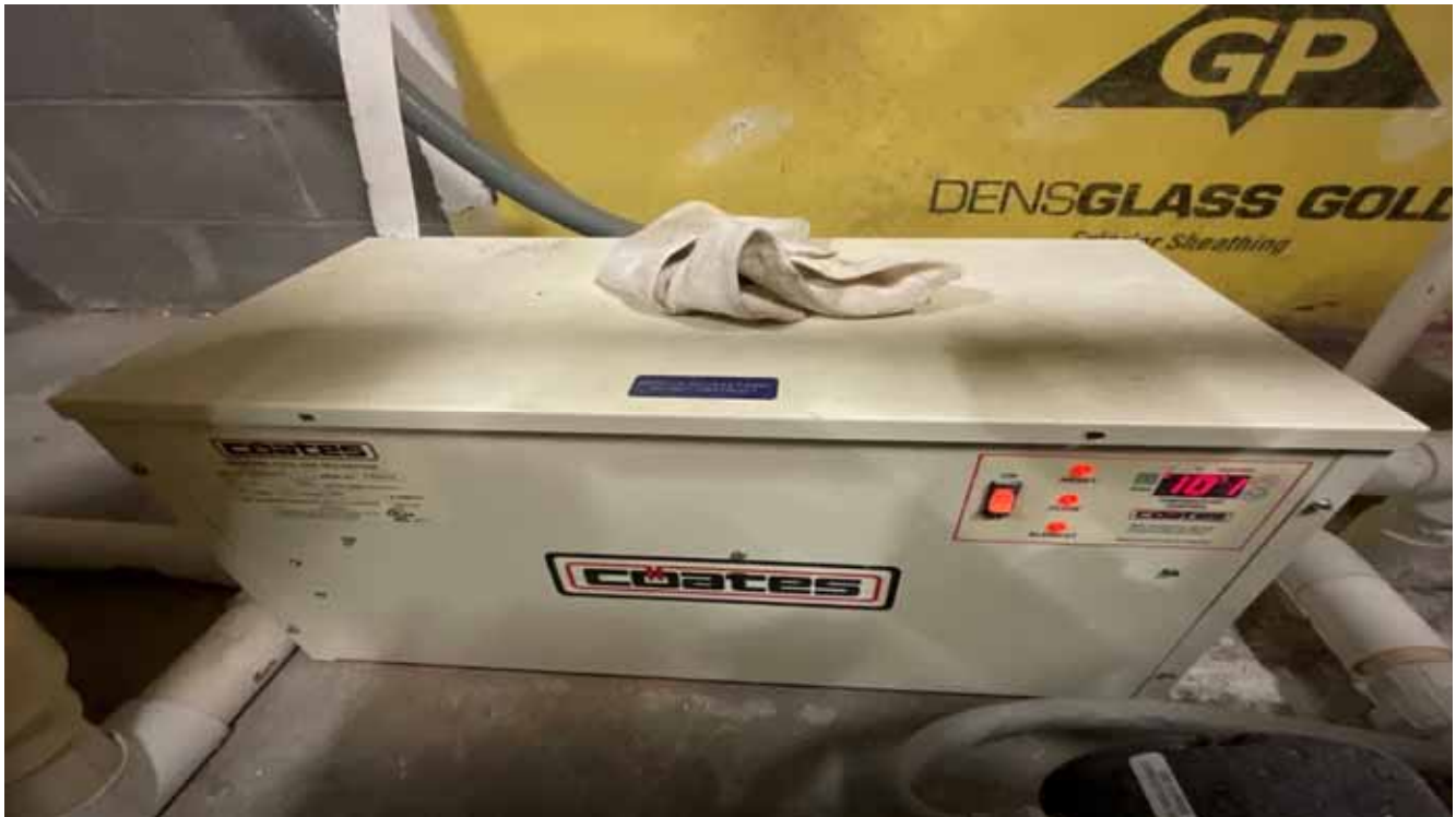
Indoor Pool Equipment, Heater
