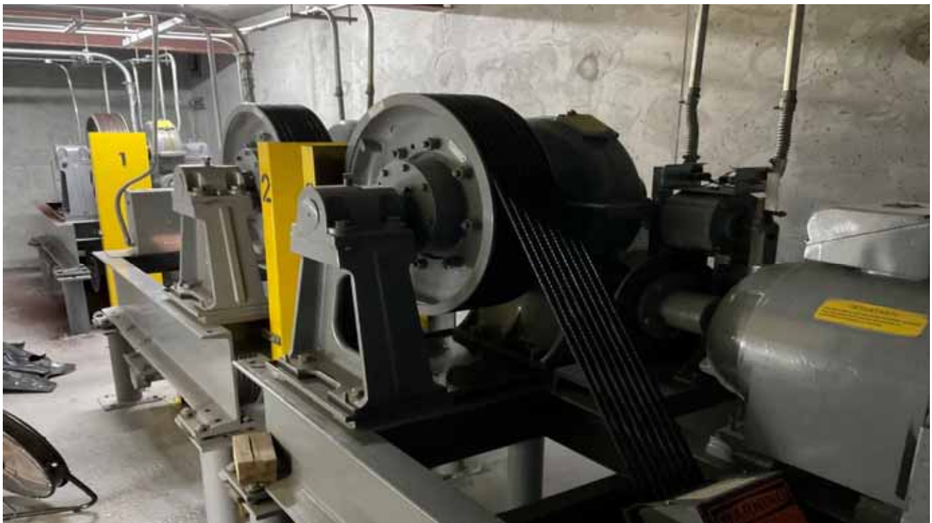
Condo Bldg Elevator Equipment
