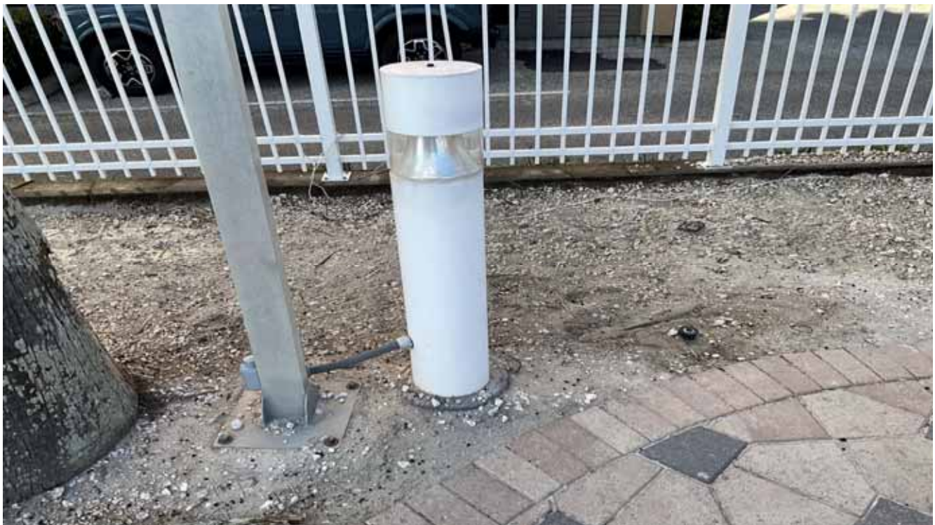
South Pool Area Light Bollard
