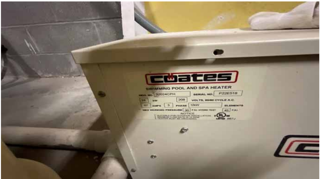
Indoor Pool Equipment, Heater
