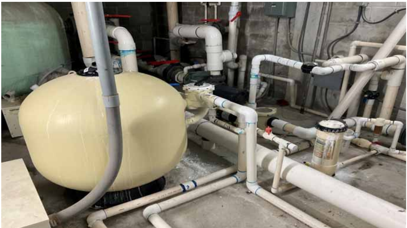
South Pool and Spa Equipment
