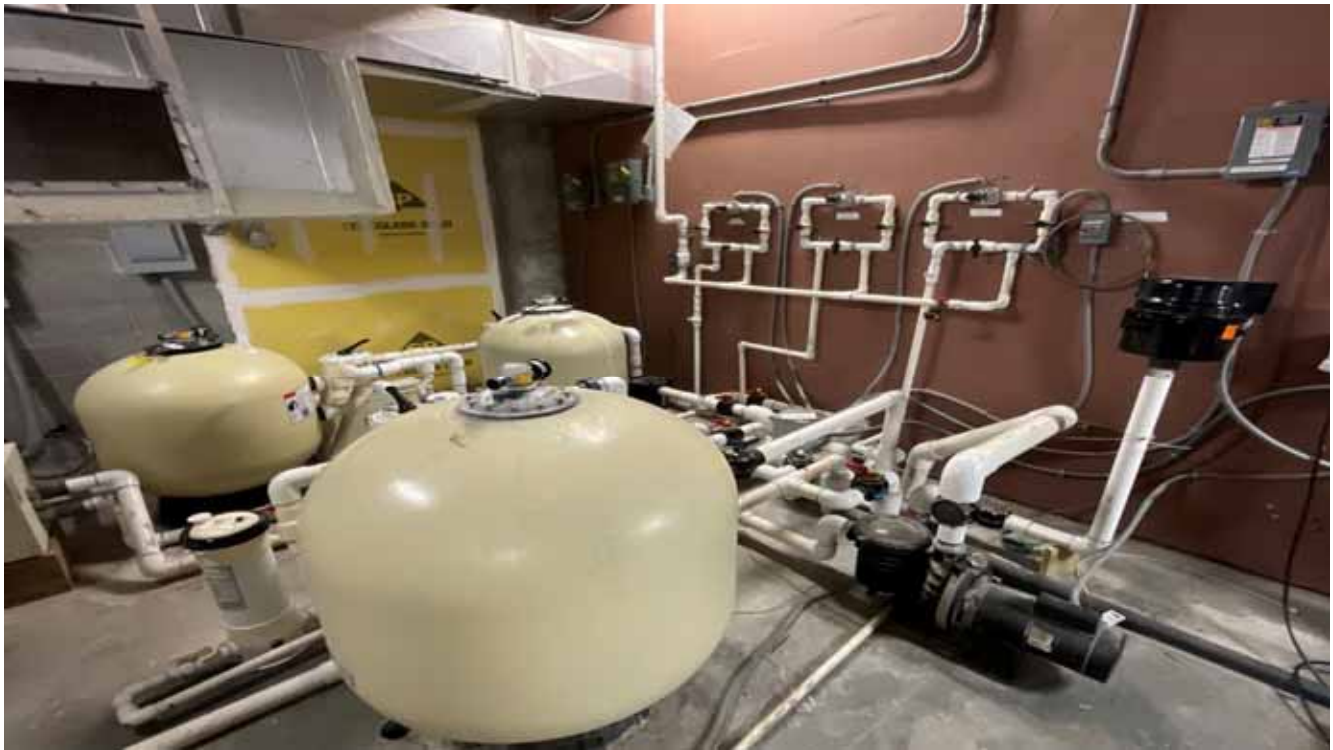
North Pool and Spa Equipment
