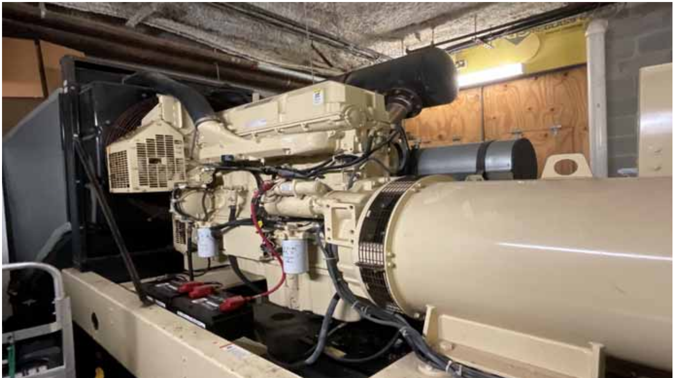
Condo Bldg Generator
