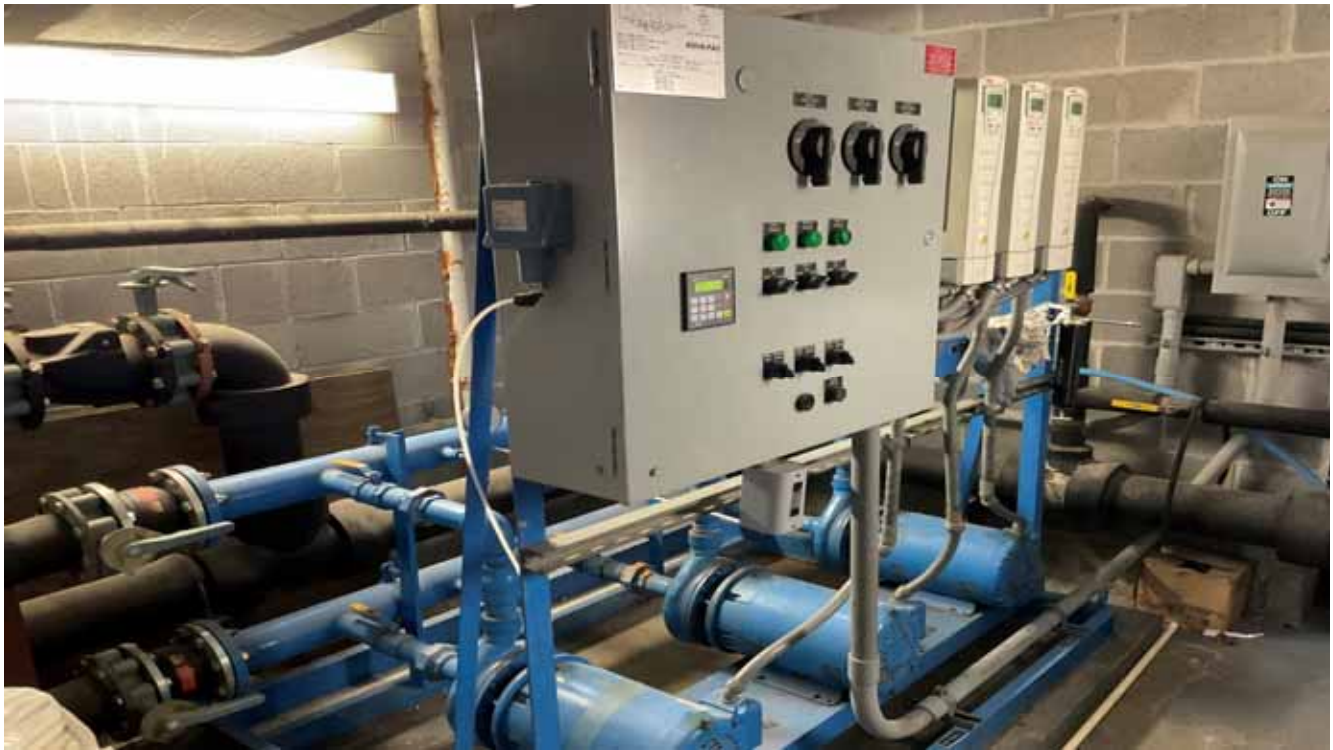
Condo Bldg Domestic Water Pump System
