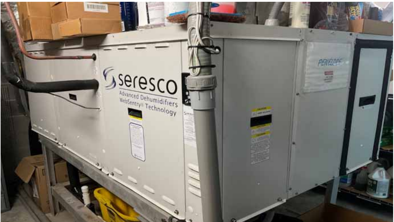
Indoor Pool Area Dehumidifier
