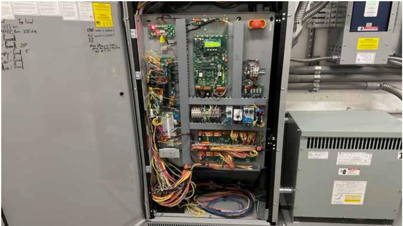
Condo Bldg Elevator Equipment
