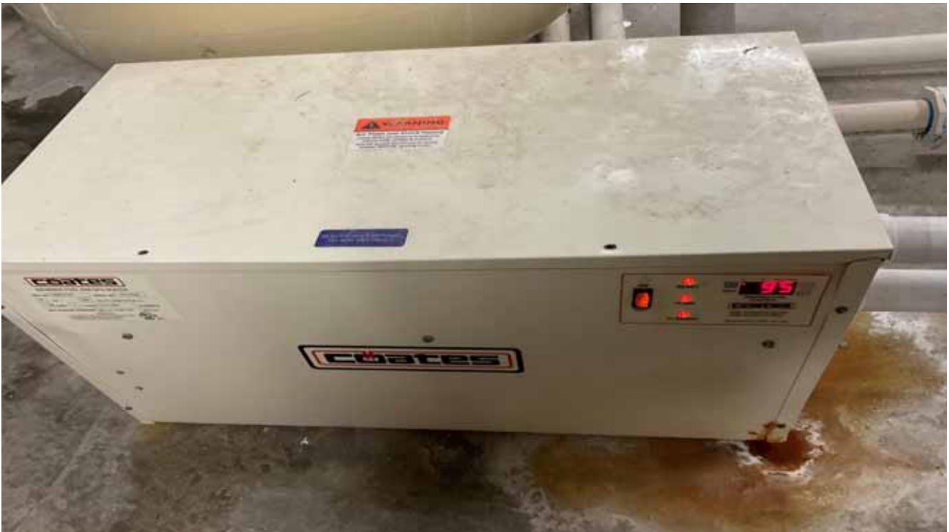
South Spa Equipment, Heater
