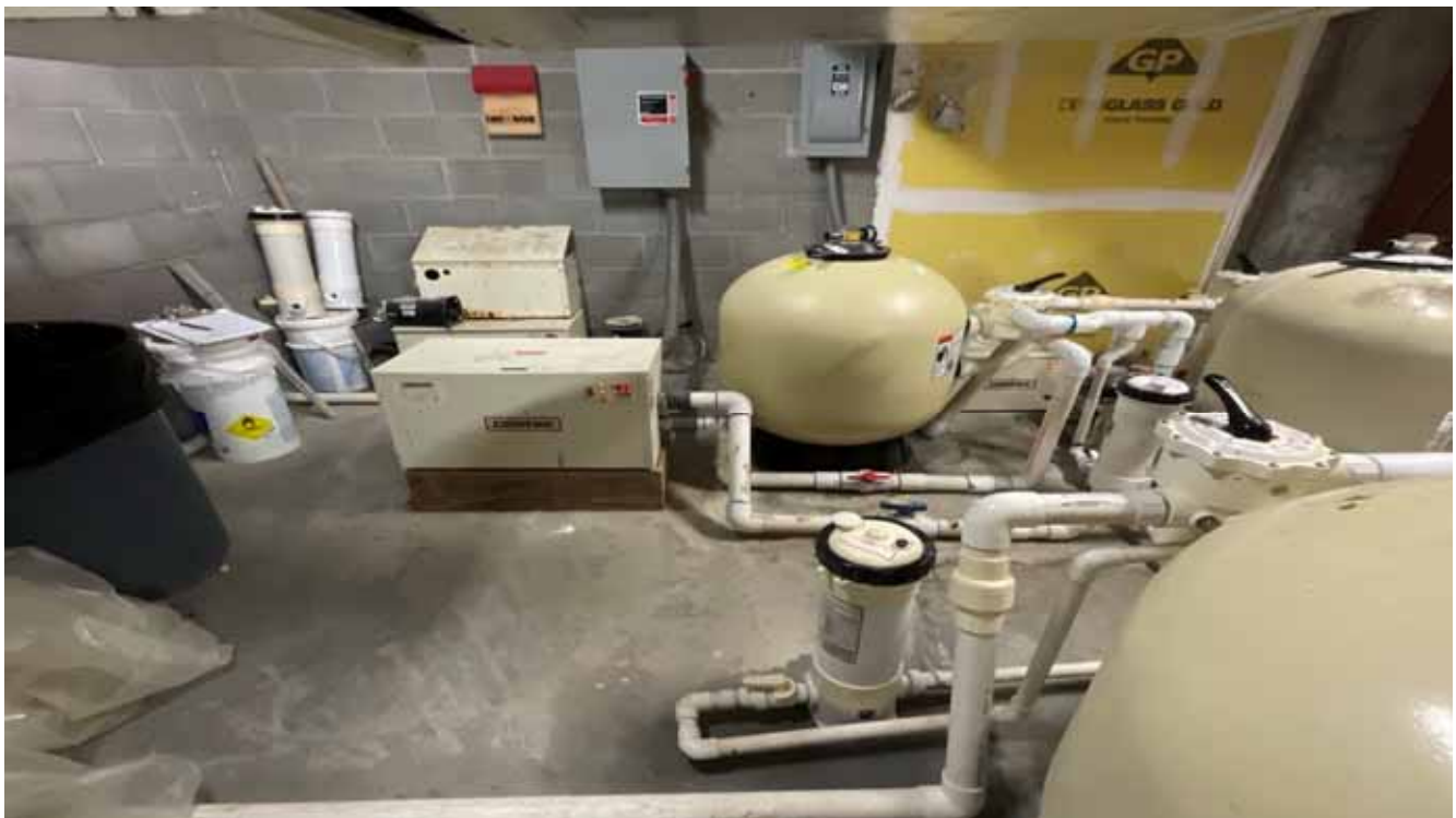
North Pool and Spa Equipment
