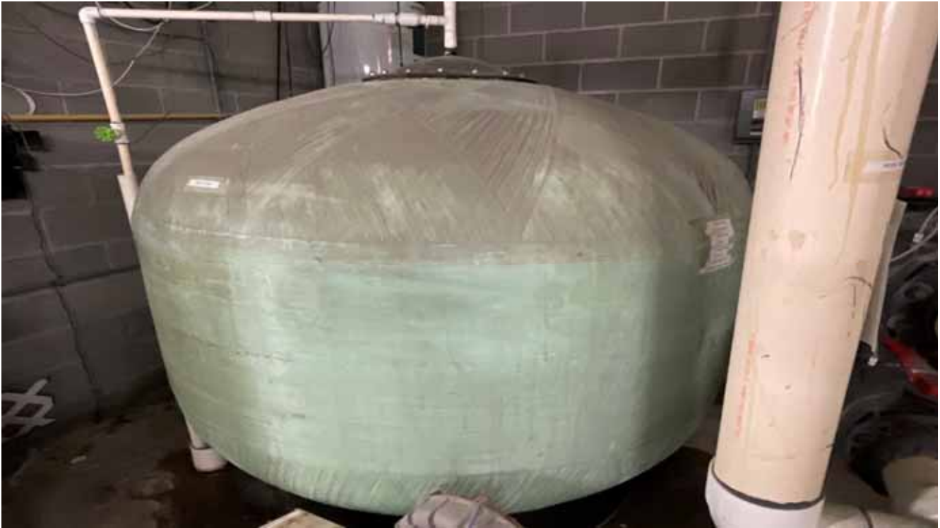
South Pool Equipment
