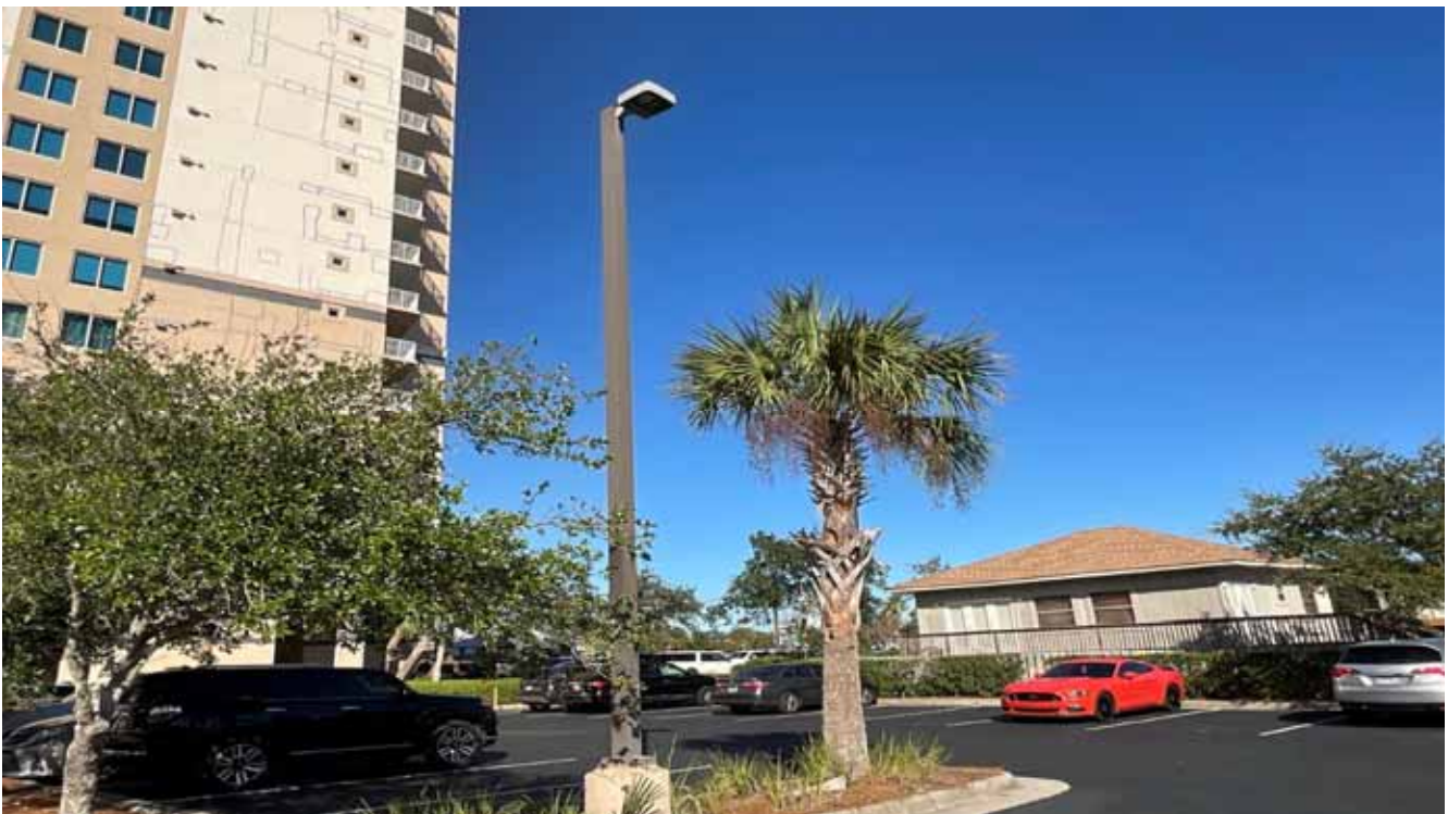
Light Pole - Parking Lot
