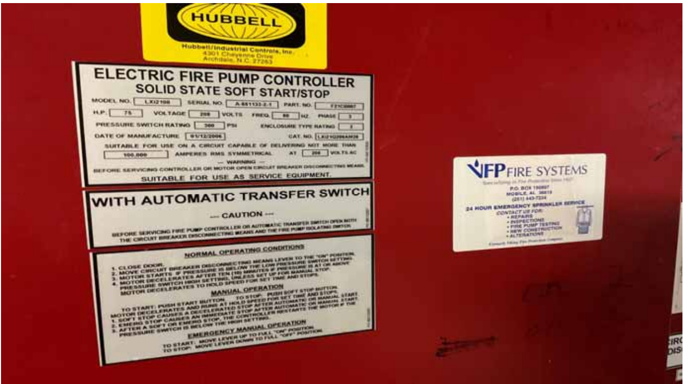
Condo Bldg Fire Pump Controller
