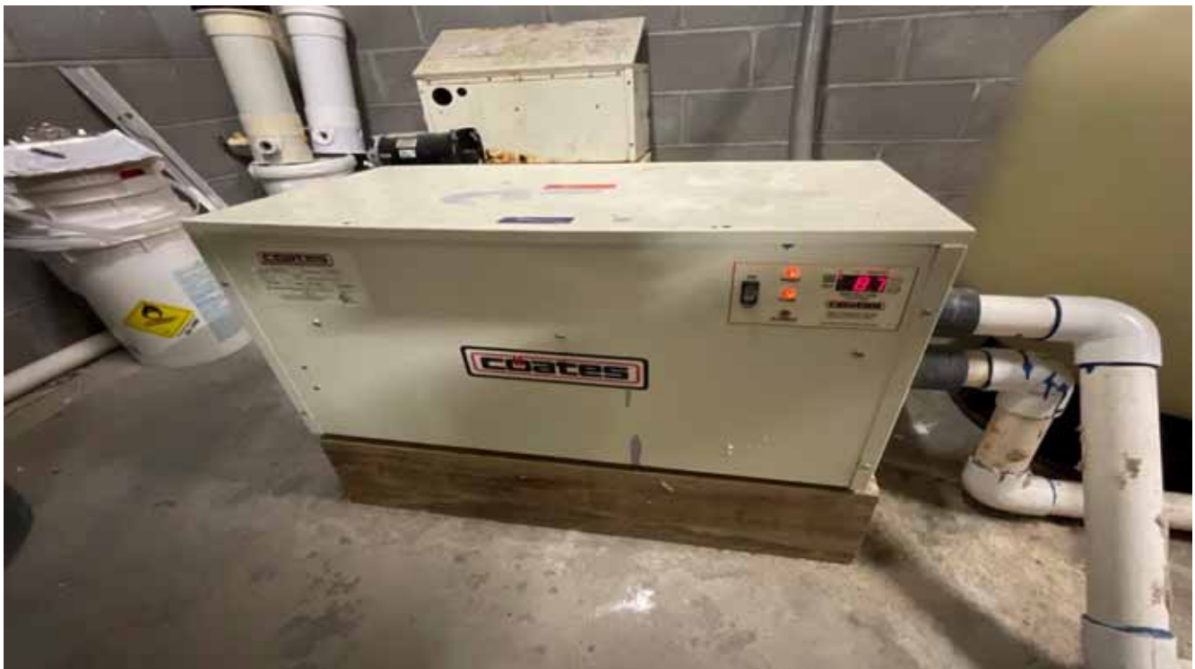
North Pool Equipment, Heater
