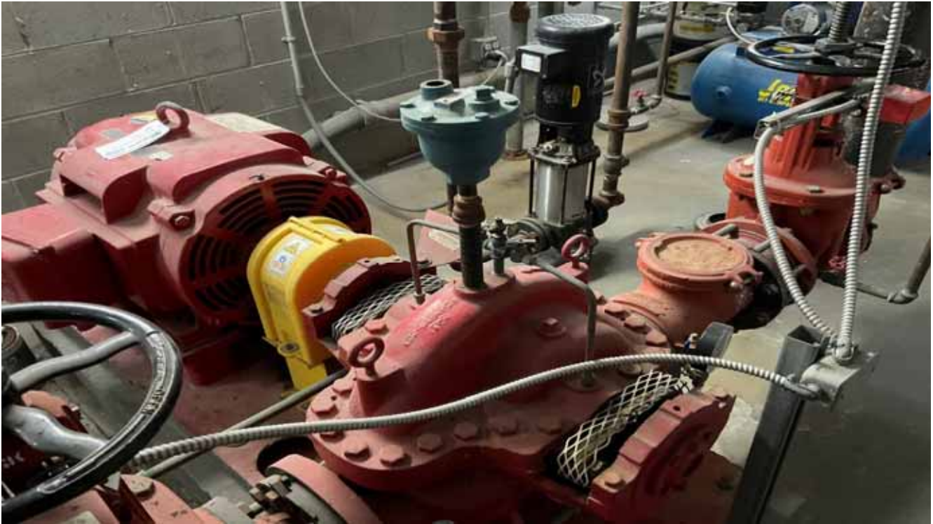
Condo Bldg Fire Pump
