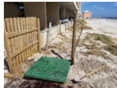
From scrap lumber and the remains of the ruined boardwalk, we built a wash station.
