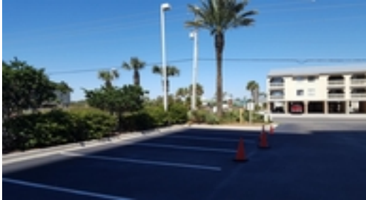
The last parking spaces have been sealed and striped where the elevator construction trailer rested.
